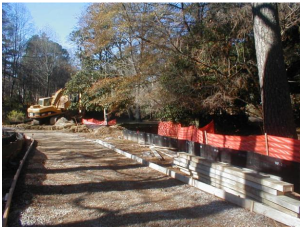
Construction near the Collier Road bridge over Tanyard Creek. One of the existing Battle of Peachtree Creek plaques is in the background, just to the left of the tree.
